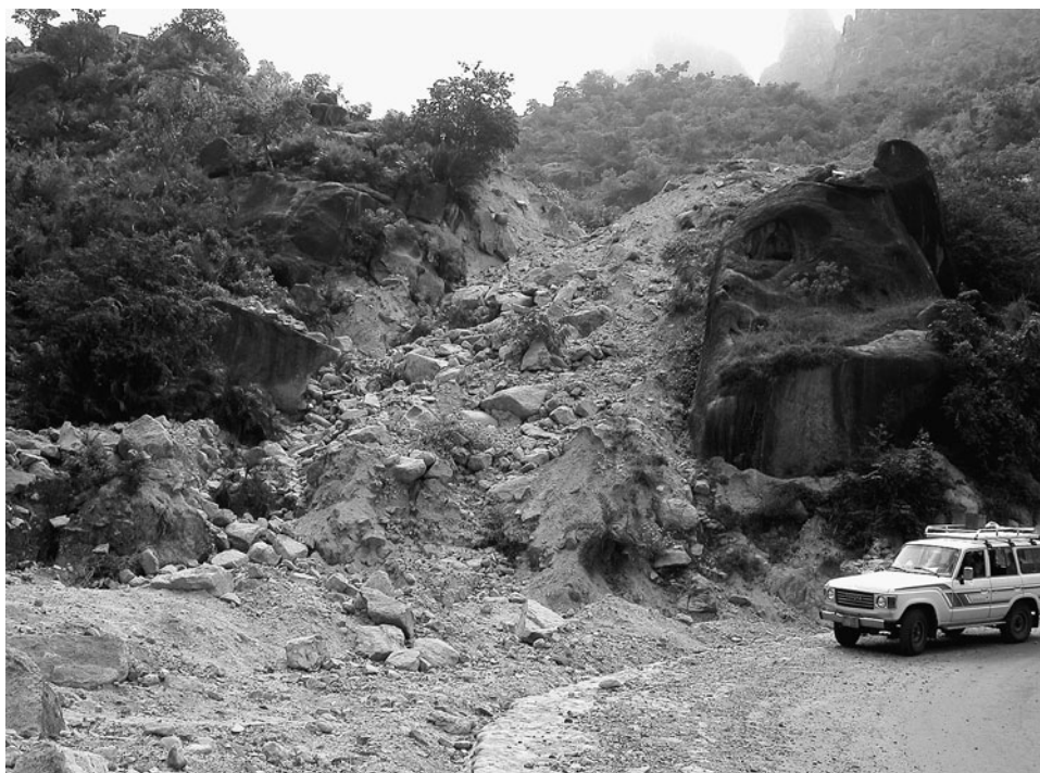
FIG. 4. An example of the erosion alongside the new road.
